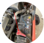
Forklift power supply
